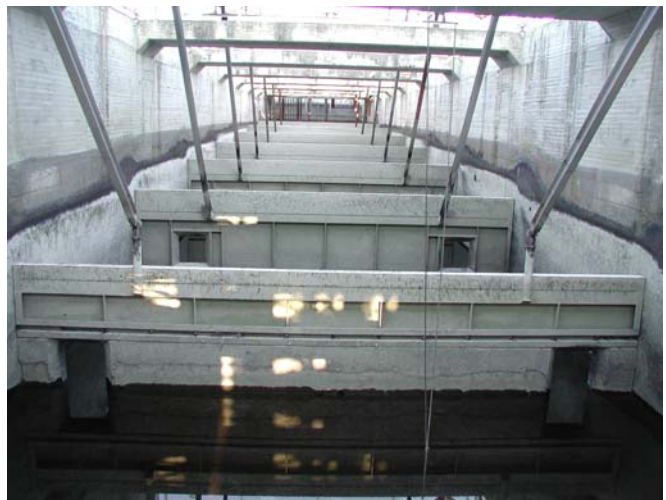
McNary Tilting Weir Gates
